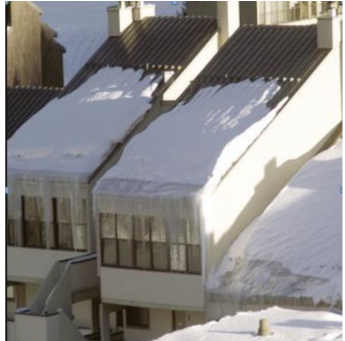
Figure 6B: Ice dams create unintentional snow retention
